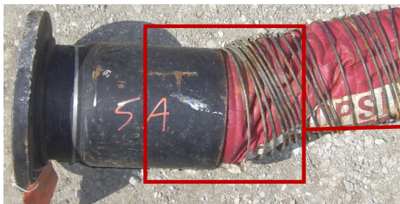
Outer wire displaced
