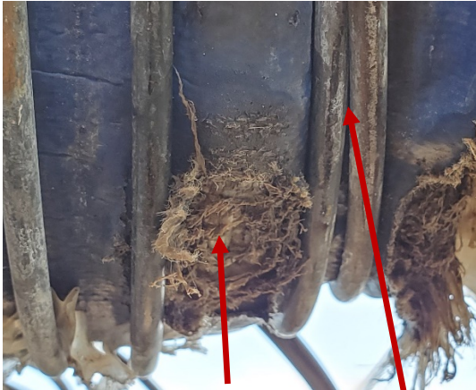
Cover damage well into the reinforcement along with wire movement
